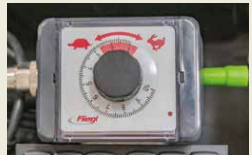
Electrical potentiometer with feed rate adjustment on control panel
